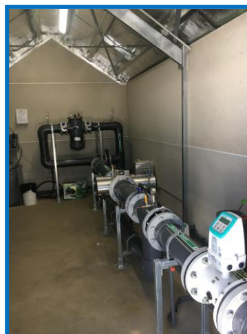
Interior of High Level Water Treatment Plant Building
