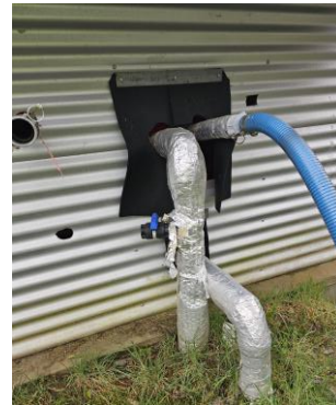
Monitoring of pumps and consumption, and protection of pipes to avoid cracking is critical.
