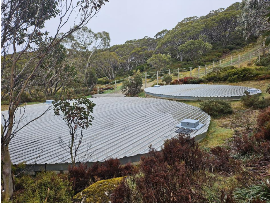
Figure 6. Raw water storage tanks
