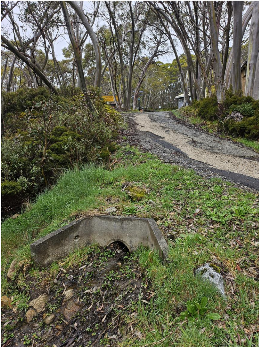
Figure 9. Local stormwater infrastructure at Mt Baw Baw
