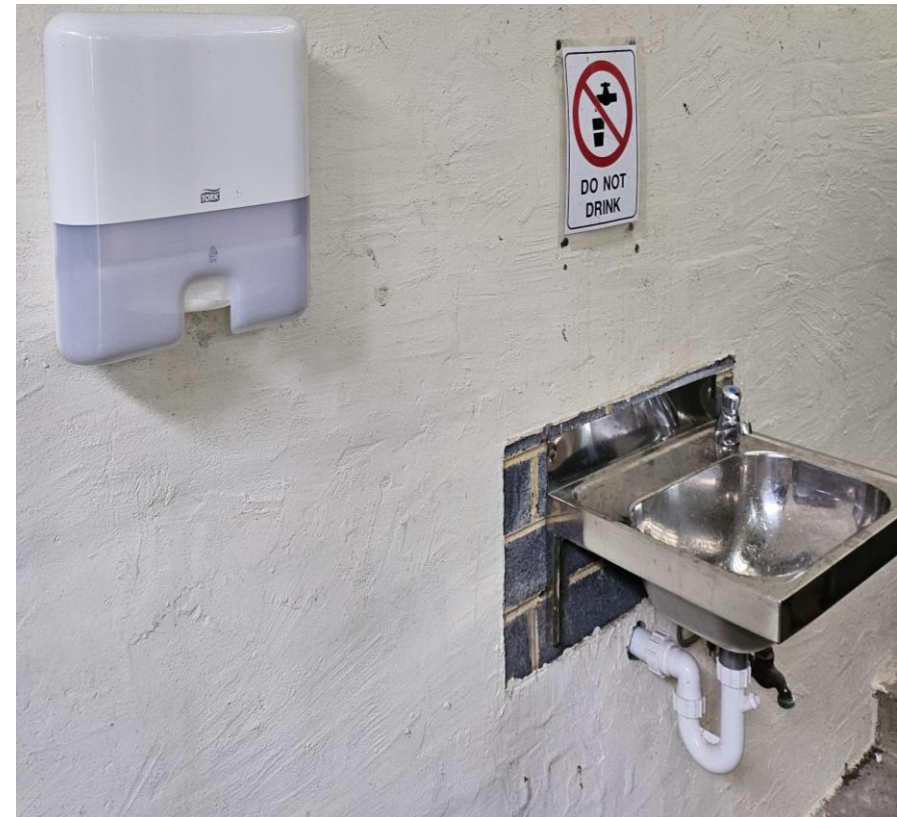
Figure 8. Photo of tank water outlets in public toilets
