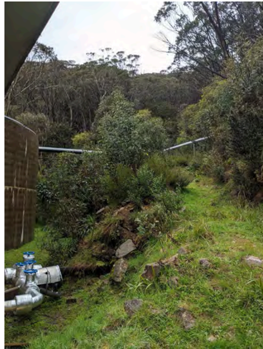
Figure 2 Location of Boggy Creek 1 PU 1 – follow grassed path past the overhead PVC pipe behind the tank
