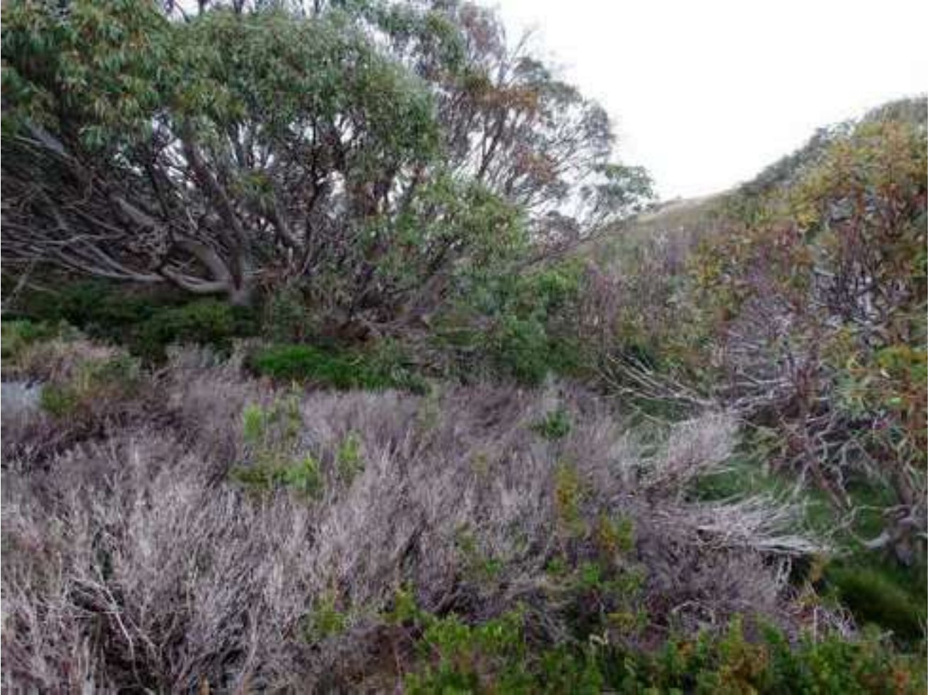
Photo 5 Dieback of non-bog-dependent flora near southern boundary of Bog 4.2 (Location D11/D14; IY4; 28 February 2023)
