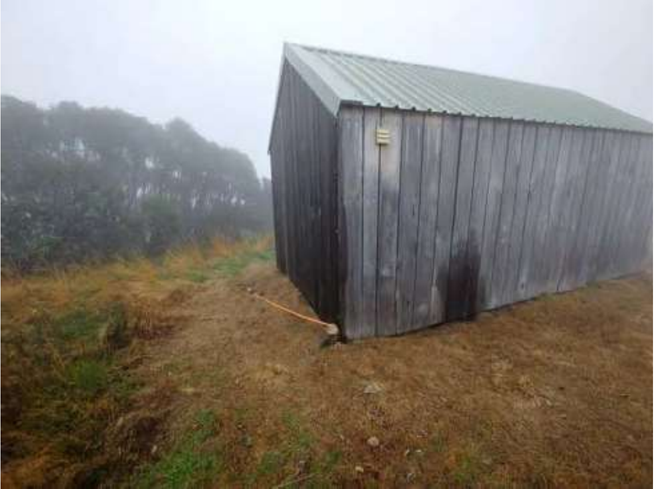
Photo 2 Discharge of water from Baldy Turrent pump house, upslope of Bog 1 (IY4; 28 April 2023)
