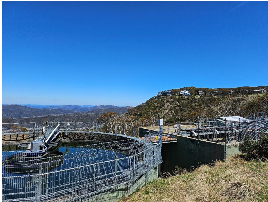
Figure 9. Wastewater treatment along Davenport Drive (Source: Wave Consulting Australia)
