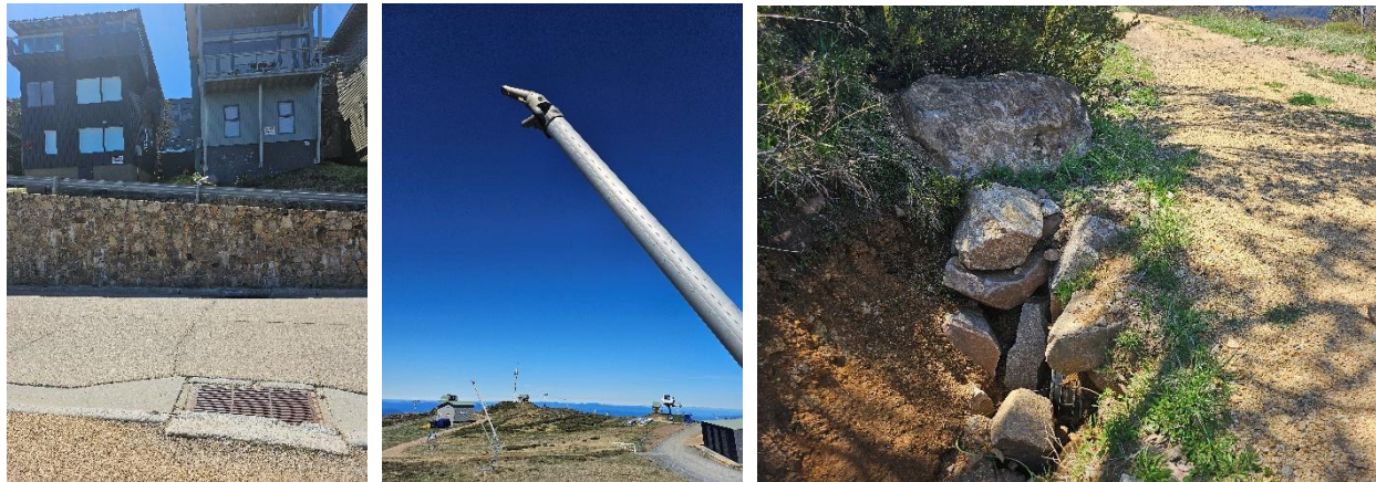
Retrofitting water efficiency, monitoring, metering and leak detection can be difficult, but has the potential to offset or defer additional water supplies and/or infrastructure needs.
