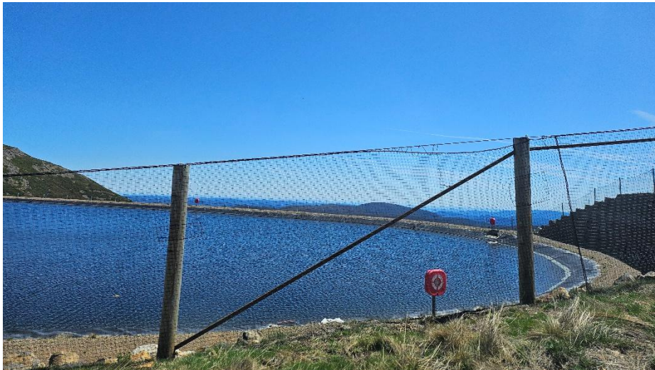
Figure 7. The 100 ML Boggy Creek Reservoir water storage reservoir at Mt Buller (opened 2020).
